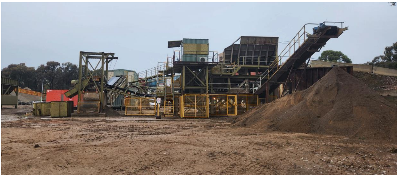
Figure 6: Discharge end of plant
