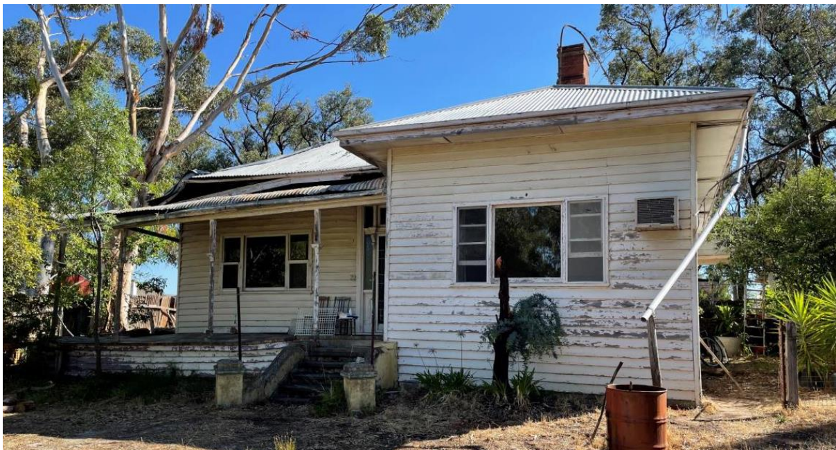
Figure 5: The dwelling (after damage)
