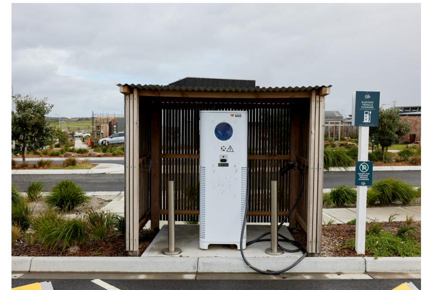
Electric vehicle charging station at The Cape development. Photography by Kim Landy
